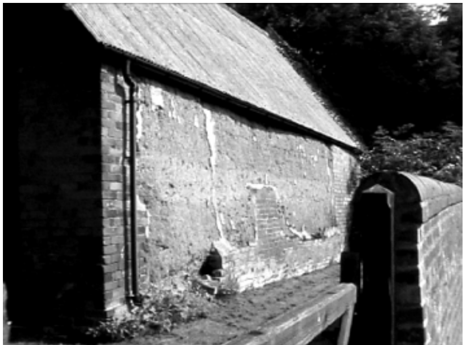
MUD BARN WALL AND TIMBER BEAM INCORPORATED INTO A MODERN STRUCTURE AT GREAT BOWDEN JULY 2000.
